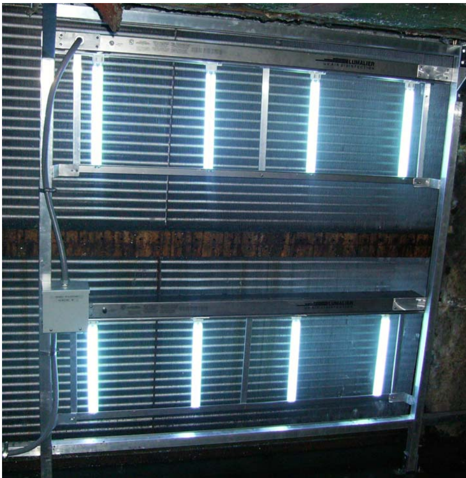
UV germicidal energy applied to coils disinfects the moving airstream and eliminates biological growth that can 'seed' the air with mold. Germicidal energy also reduces energy costs by increasing heat transfer and air flow
